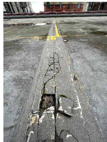
Fig. 14 – Damaged seal over joint
