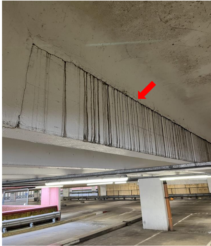
Fig. 5 – Typical crack at original construction joint, along top of rib
