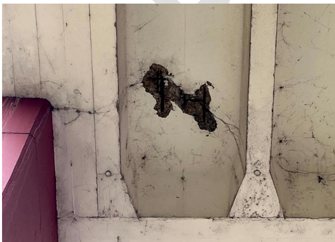
Fig. 9 – Transverse crack, slab underside
