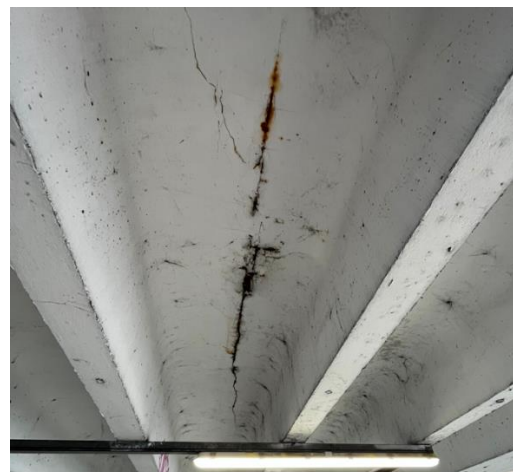
Fig. 10 – Longitudinal crack, slab underside
